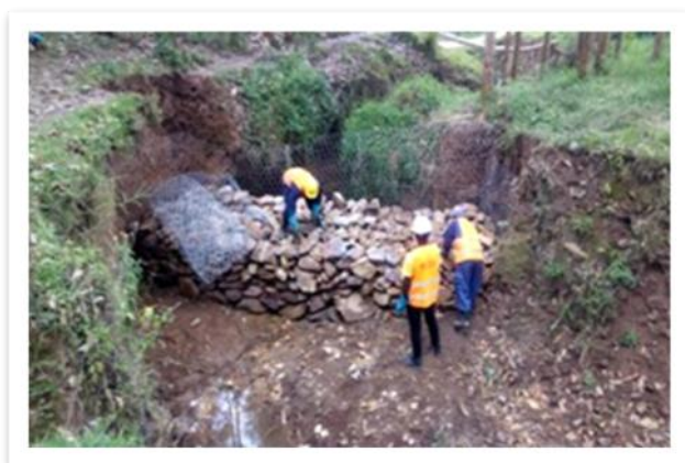
Kaato GFS reservoir tank of 20000 litres
